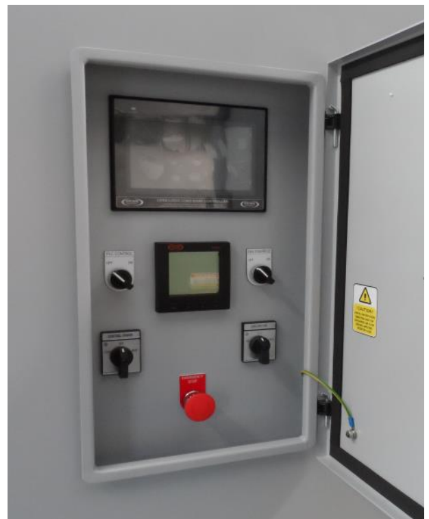
Control panel with 7" HMI and digital power meter
